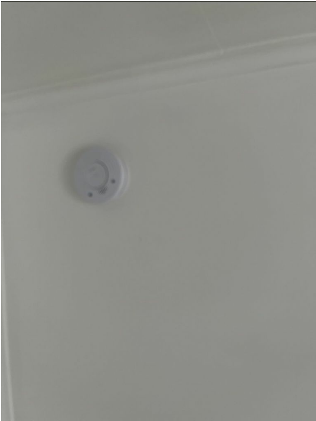
1. Smoke alarms 14/08/25 at 11:47 AM
